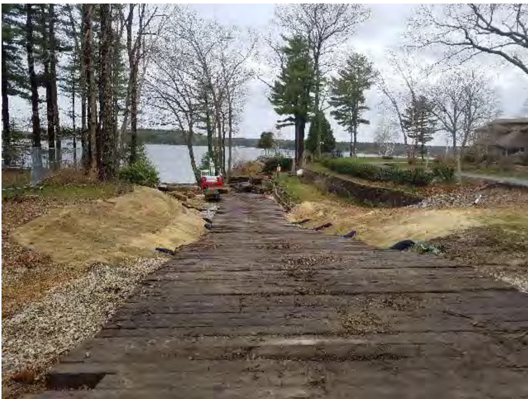
Fig 14: Blu Roc installed timber mat road to access the intertidal zone at Gundalow landing/east side of the Bay. Viewing west. (04-28-20).
