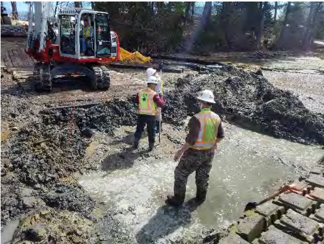
Fig 22: Blu Roc excavating tidal flat to bury concrete blocks over cables at Gundalow landing/east side of the Bay. Viewing southeast. (04-29-20).
