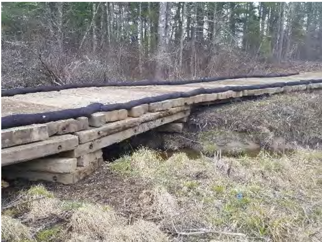
Fig 6: Timber mat bridge over stream DS60 in wetland DW58. Between Strs. 43-44. Viewing southeast. (04-24-20).
