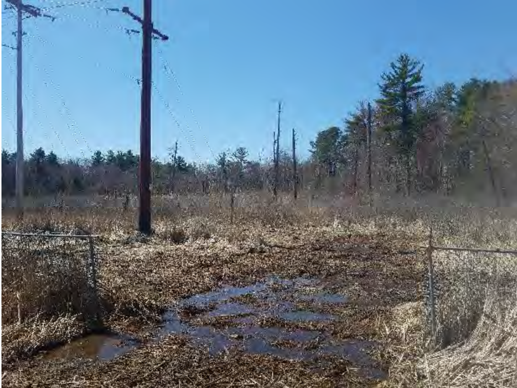
Fig 3: Str. 128 pole set and timber mats removed in wetland NW1. Viewing south (04-23-20).
