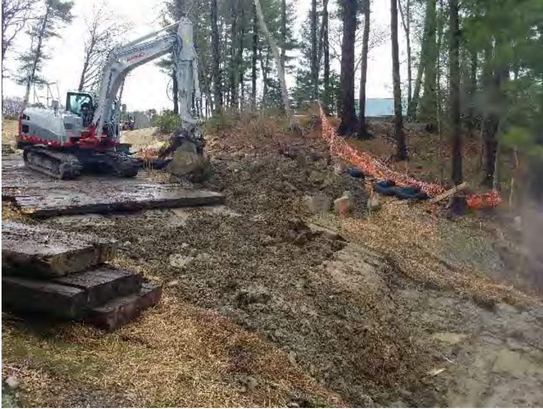
Fig 15: Blu Roc installing timber mat access road to access the intertidal zone at Gundalow landing/east side of the Bay. Viewing west. (04-28-20).
