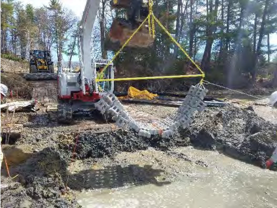
Fig 23: Blu Roc installing concrete blocks for submarine cable protection at Gundalow landing/east side of the Bay. Viewing southeast. (04-29-20).
